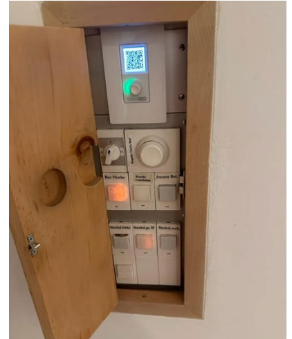
AtlasIED C-ZSV ZONE, SOURCE, AND VOLUME WALL CONTROLLERS IN THE LOUNGE, BREAKFAST ROOM, AND VIVANDA RESTAURANT TO CHANGE MUSIC AND VOLUME.
